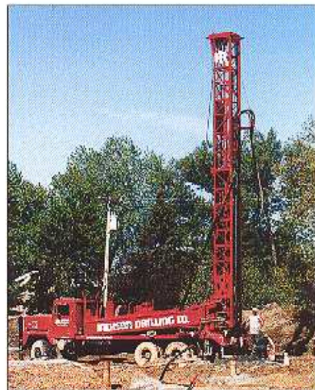
The geothermal HVAC system being installed at the Immaculate Heart of Mary Motherhouse requires drilling 232 bore holes, each 450 feet deep, on the 280-acre campus in Monroe.
