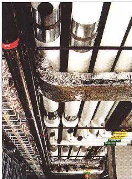
GEM Industrial is filling the ceiling of the lower level of the Immaculate Heart of Mary Motherhouse with racking, piping and ductwork for the electrical and mechanical renovation of 240 residential units and offices. A geothermal heating and cooling system is being installed.
